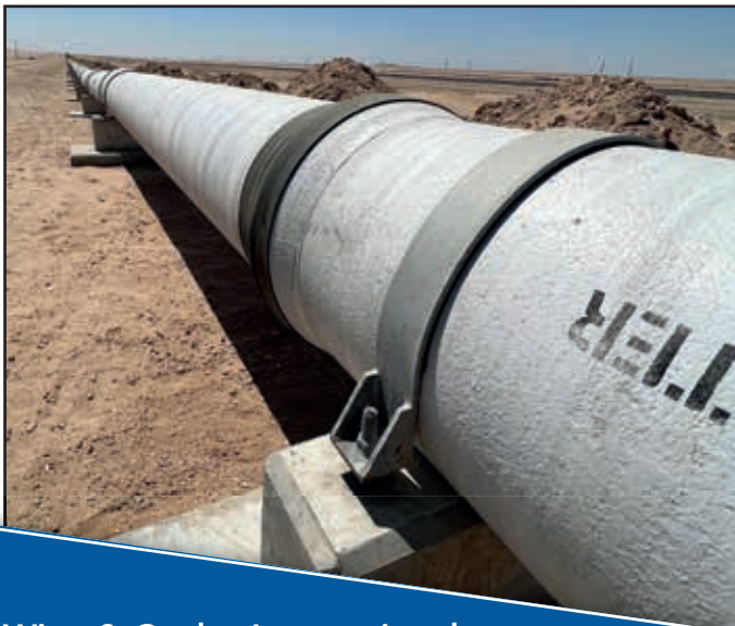
Above ground pipe with threaded round bar and strapping securing pipe.
