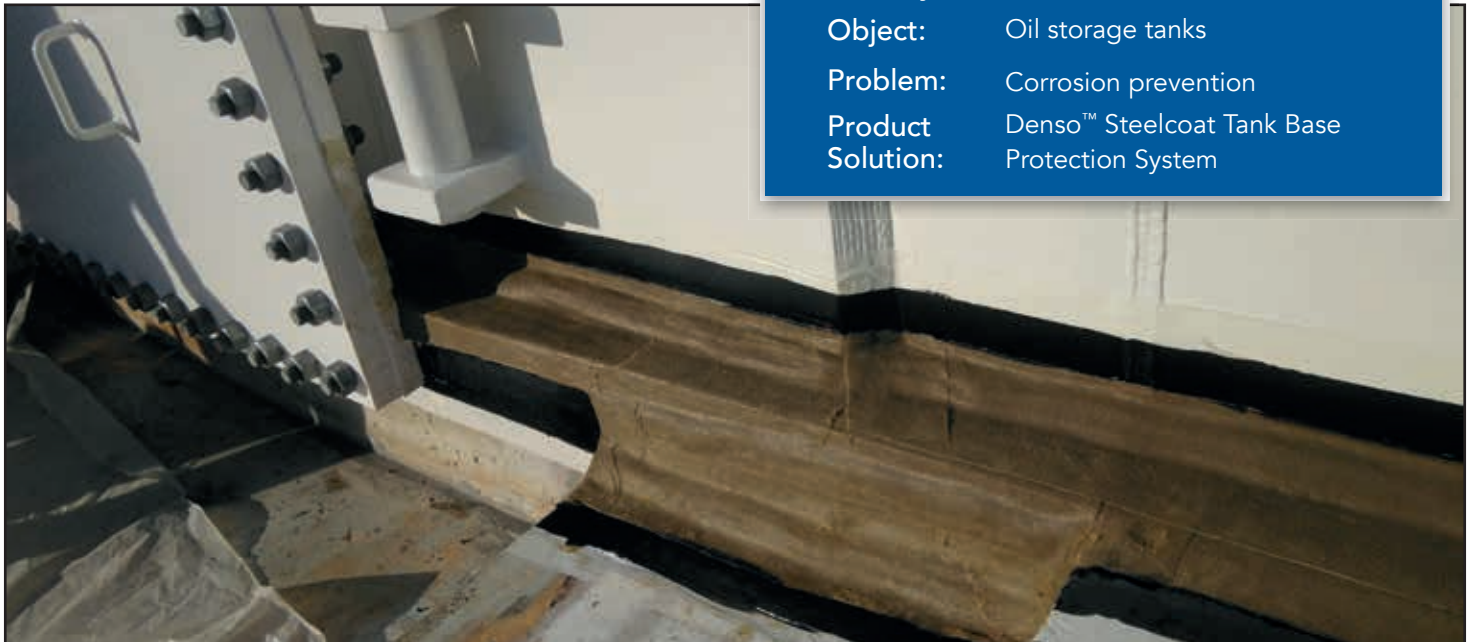
Above: After cleaning the substrate around the berm seal area and coating it with Denso™ Hi-Tack Primer, any voids or internal angles are filled with Densyl™ Mastic to form a smooth profile before applying the layer of Denso™ Hi-Tack Tape. Then Denso Primer D™ is applied to the area immediately around the Denso Hi-Tack Tape in a minimum 50mm strip and allowed to dry (Primer D is the black area in the picture).
