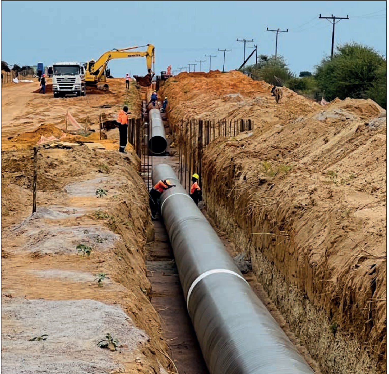
Excavator backfilling once the pipeline has been installed and inspected for any damages..
