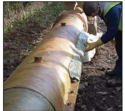
Above: Densyl Mastic being applied to profile the half shell bolts prior to wrapping with tape.
