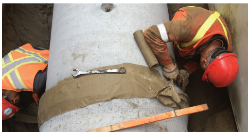
Workers sealing the Denso LT Tape by hand, ensuring that all air is pushed out and seams are closed, providing a water tight seal.
