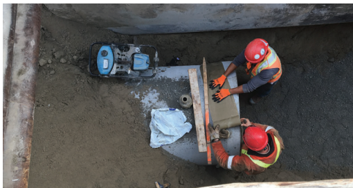
A section of the 1 metre diameter wastewater concrete piping installation being prepped for water infiltration protection with Denso LT Tape.
