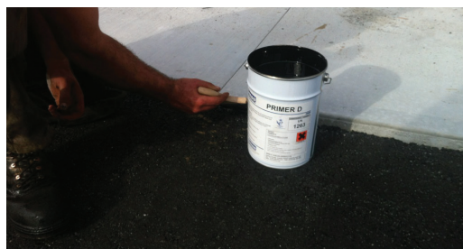
Denso Primer D, a bitumen primer, is applied to the concrete prior to installing the DensoBand™ along the joint.
