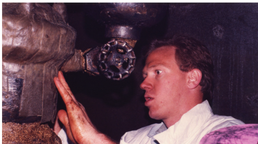
Over 100 valves and fittings were protected with the Denso Petrolatum Tape System.
