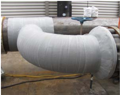
Cooling tower piping, tank bases and pipe under thermal insulation.
