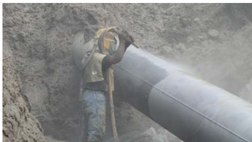
Abrasive blasting to a near white metal finish before applying the Protal 7200.
