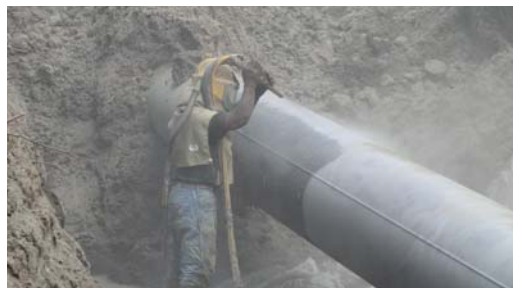
Abrasive blasting to a near white metal finish before applying the Protal 7200.
