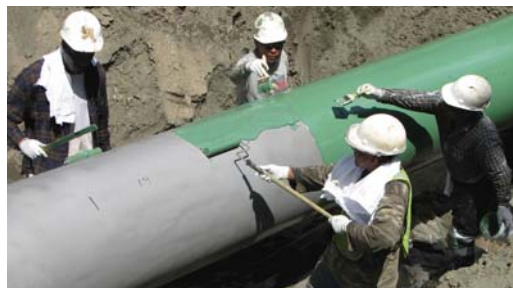
Once mixed and ready for use, the Protal 7200 is easily applied to 50' sections of pipe.
