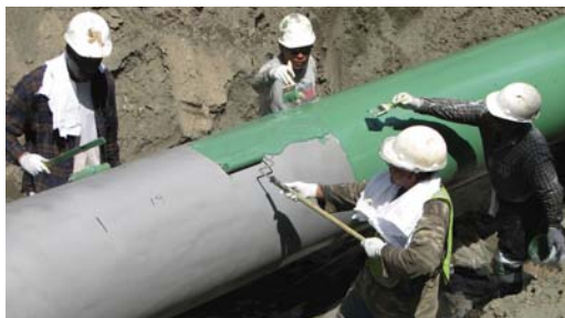
Once mixed and ready for use, the Protal 7200 is easily applied to 50' sections of pipe.
