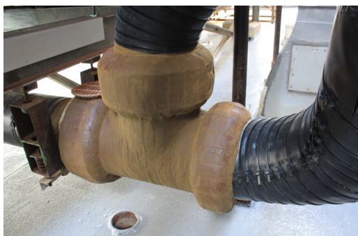
Piping protected with an HDPE Outerwrap and Smartband Strapping system.
