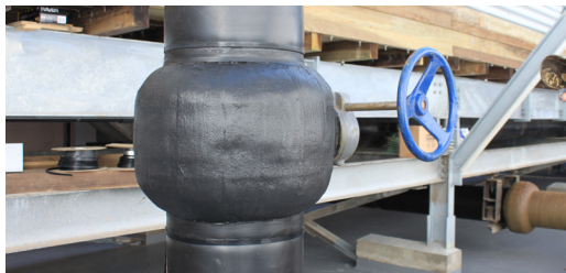
Weathershield 15 brushed applied onto Densyl Tape protecting a valve flanged as a top coat.
