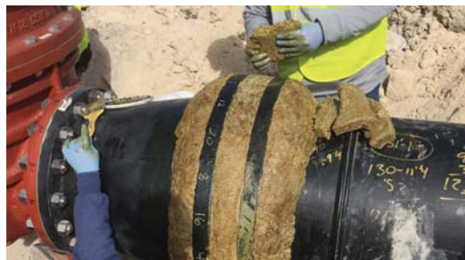
Application of the Denso Profiling Mastic creating a smooth profile for the Densyl Tape.
