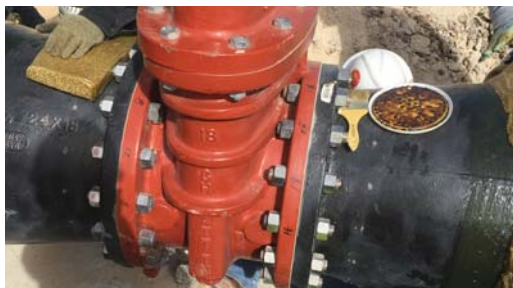
Surface prepared in accordance to SSPC SP-2/ SSPC SP-3 prior to application of the Denso Paste.
