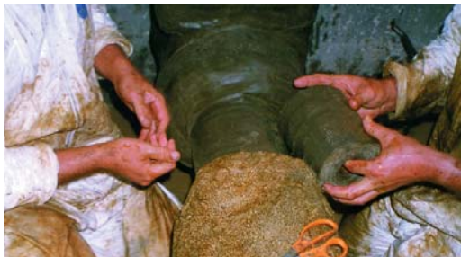
Densyl Tape is applied over the smooth contours of the Denso Profiling Mastic.
