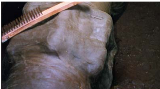
Completed application of one many valves and meters with Denso Petrolatum Tape System.
