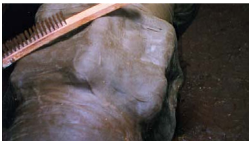
Completed application of one many valves and meters with Denso Petrolatum Tape System.
