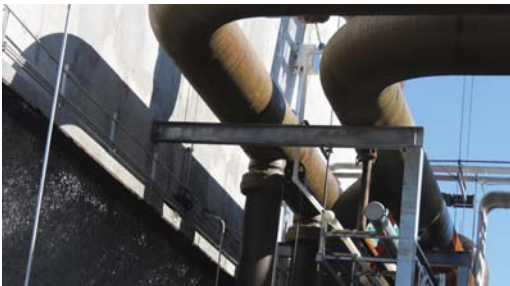
Denso Paste S105 and Densyl Tape applied to all straight pipe and bends.
