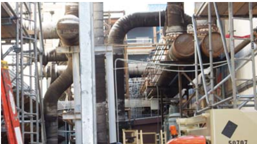
Denso Petrolatum Tape System applied 30 years ago to the old cooling tower and still performing well.
