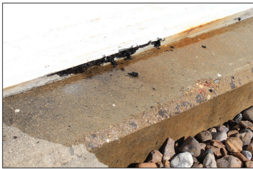
Tank caulk used as a sealant has a tendency to crack and absorb water over time.
