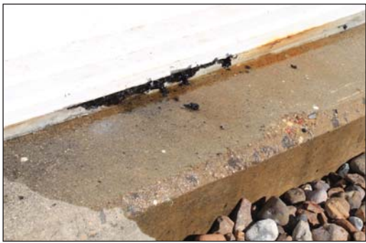
Tank caulk used as a sealant has a tendency to crack and absorb water over time.
