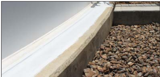
Finished tank with Denso Weathershield 55 applied as a top coat completing the system.
