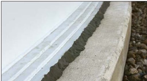
Tank plinth area seal with Densyl Mastic to prevent moisture from entering.
