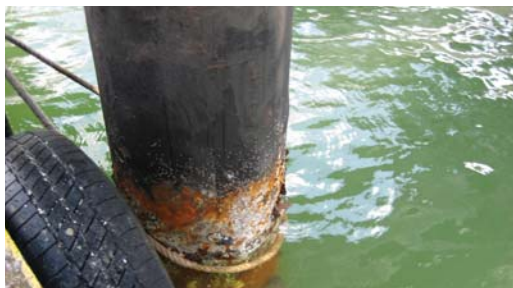
Severe corrosion of pile prior to cleaning.
