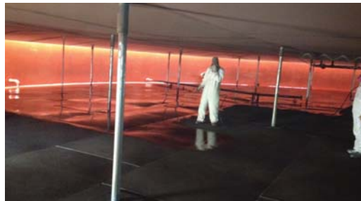
400 primer on a side wall and floor on a diesel tank in Texas.
