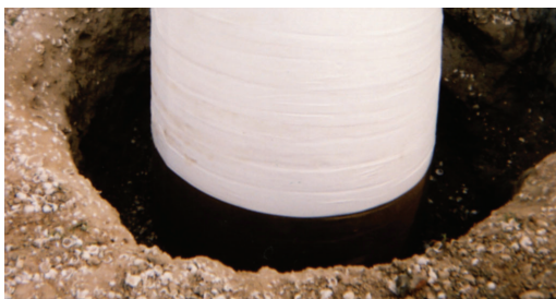
Pipeline covered with Denso Glass Outerwrap, which is resistant to water, acid, salts and soil organics.
