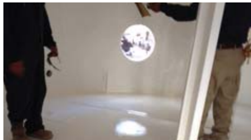
Holiday testing the Archco 453HT coating and confirming it was pin-hole free.
