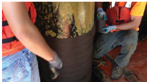
Installation of Denso S105 Paste and Densyl Tape to a 24" steel pile.
