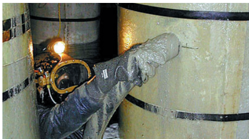
Concrete is pumped into the annulus space between the jacket and timber pile.
