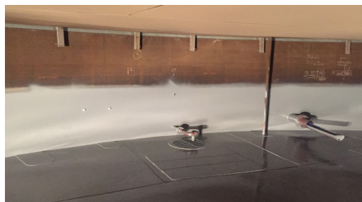
Fully cured Archco 476P lining allowing the tank to return to service within 8 hours.
