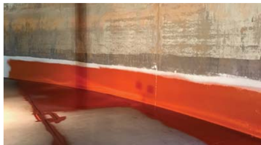
Archco 400 primer being applied to the blasted floor and side walls of the tank.
