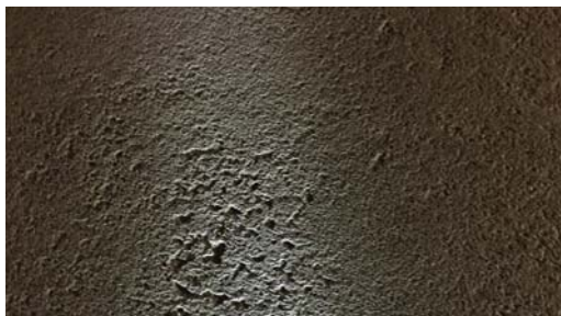
Heavy pitted floor.
