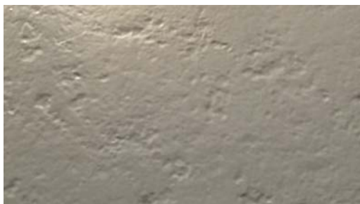
Heavy pitted floor with 401/476 pinhole free.
