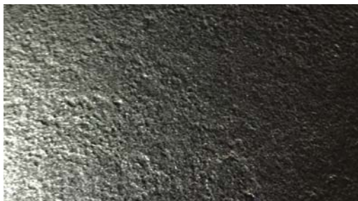
Heavy pitted floor with 401 sealer.
