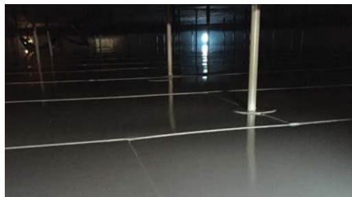
Finished Archco 400/400HB tank lining.
