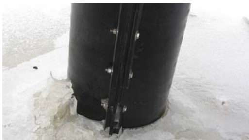
SeaShield Series 2000HD protecting a steel pile during winter ice build up.
