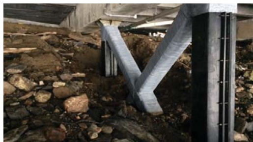
Steel cross beams protected with Denso Glass Outerwrap UV in lieu of the 80 mil HDPE Outercovers.
