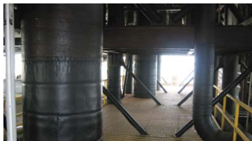
Phase 2 - installation of Densyl Tape, Denso Hi-Tack Tape and Denso Utility Tape.
