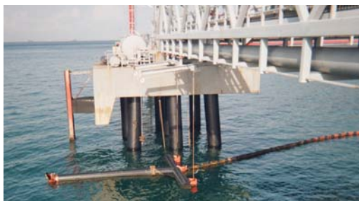
SeaShield Series 2000HD System installed on the pilings at the Decal Panama.
