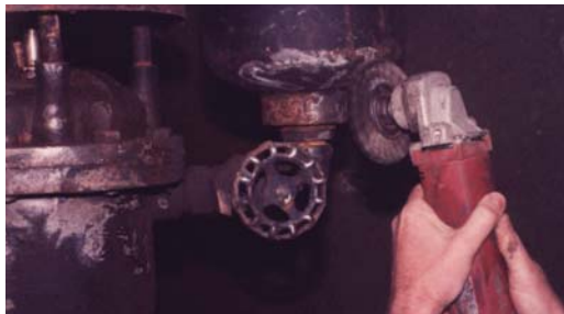
Simple hand cleaning (SSPC-SP-2 or SP-3) is all that is required for surface preparation.
