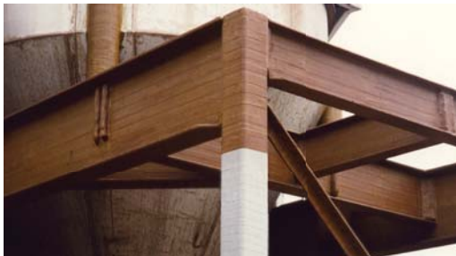
Denso Hi-Tack Tape and Denso Color Tape used to protect the steel head frame from corrosive salts.
