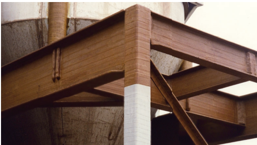
Denso Hi-Tack Tape and Denso Color Tape used to protect the steel head frame from corrosive salts.
