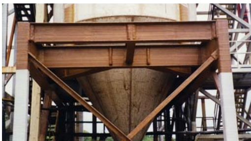
Denso Petrolatum Tape products fully protecting over 10,000 sq. ft. of steel head frame.
