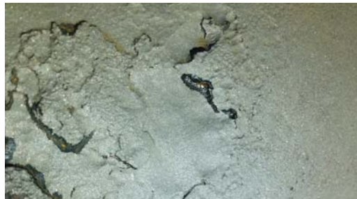
Severe corrosion and pitting was discovered when tape was removed, and the pipe was sand blasted.
