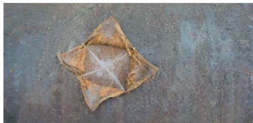
An inspection of the pipe revealed the surface underneath the tape to be in excellent condition with no corrosion.
