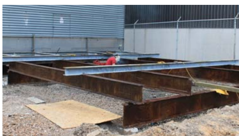
The maintenance crew completing the wrap protection system to the cooling tower frame work.
