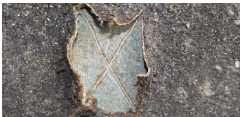
Inspection of the I-Beam, with Densyl Tape protecting since 1977, revealed the surface underneath to be in excellent condition with no corrosion.
