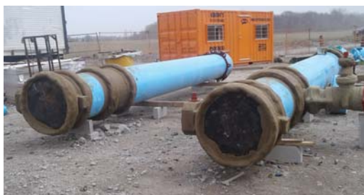
Some of the Denso Petrolatum Tape System installation was applied prior to placing in-situ.
