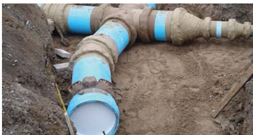
Metal valve assemblies and fittings protected with the Denso Petrolatum Tape System.
