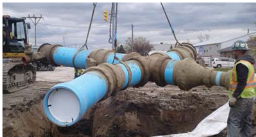
Fully corrosion protected valves using Denso Petrolatum tape being lowered for buried installation.
