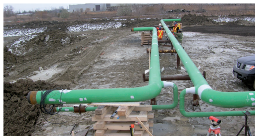
With no preheating necessary, the girth welds can easily be coated with Protal™ 7125 at temperatures of -15°C.
