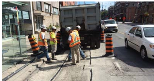
The Densoband in place along both of the vertical joint faces of the reinstatement trench.
