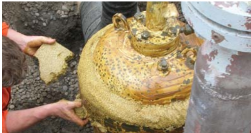
Denso Profiling Mastic is used to fill voids and smooth all irregular contours ready for wrapping with Denso LT Petrolatum Tape.
