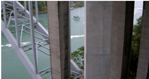
A total of 2000 liters of Denso Void Filler was used to provided anti corrosion protection for the Rainbow Bridge.
