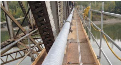
Oil pipeline suspended from a train rail bridge protected with Denso Petrolatum ColorTape.
