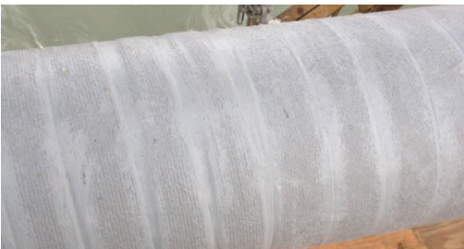
Denso ColorTape was used as corrosion prevention measure as well as a lead encapsulation means.
