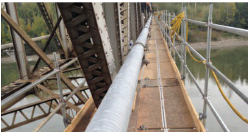
Oil pipeline suspended from a train rail bridge protected with Denso Petrolatum ColorTape.
