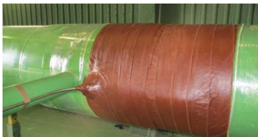
55% overlap of Denso Hotline Tape around the sensor to provide corrosion protection prior to being buried.
