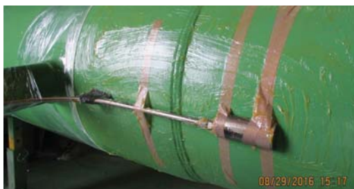
RTD Sensor attached to Protal 7200 coated pipe and a thin layer of Denso Paste HT coating the sensor.
