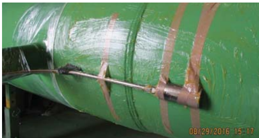
RTD Sensor attached to Protal 7200 coated pipe and a thin layer of Denso Paste HT coating the sensor.
