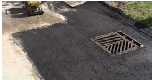
The joint is now protected from damage by water and ice for decades to come.
