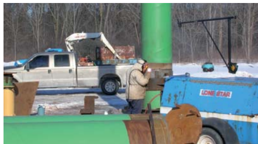
A steel air shaft is welded to a tunnel section prior to the Protal liquid epoxy coating application.
