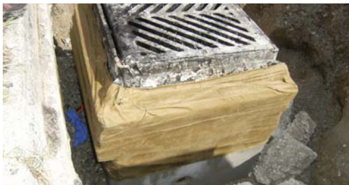
Frame and grate chamber wrapped in Denso LT Tape to prevent water corrosion.
