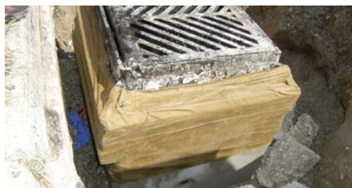
Structure, risers and frame of a catch basin quickly wrapped to prevent erosion corrosion.
