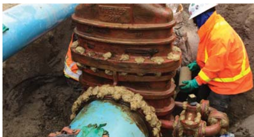
Voids and awkward angles on the valve are first filled with Denso Profiling Mastic.
