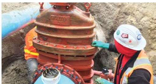
A protective coating of Denso Paste is applied by hand to provide the first layer of corrosion protection to the substrate.
