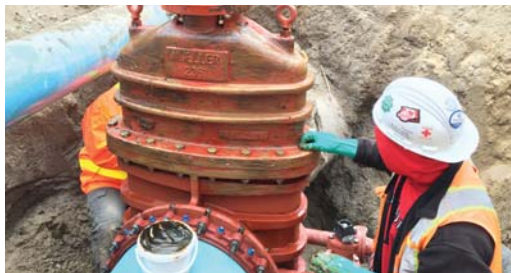
A protective coating of Denso Paste is applied by hand to provide the first layer of corrosion protection to the substrate.
