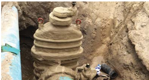
The valve is wrapped with Denso Petrolatum Tape to complete the protection.
