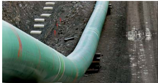
The pipelengths are welded together and the welded joint areas are then coated with Denso Protal 7200 before being buried.
