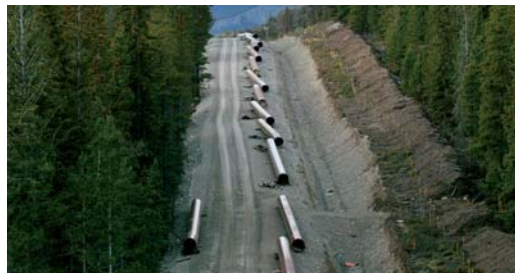
Pipe lengths awaiting Denso Protal application, mark out the route through the stunningly beautiful and environmentally sensitive Canadian National Park.
