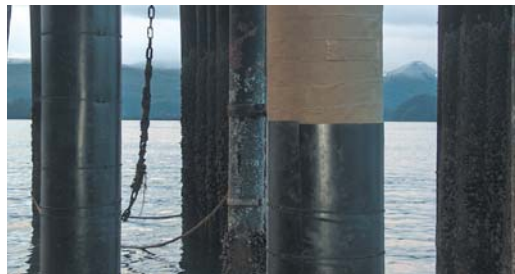
Center of picture shows Denso Marine Piling Tape protected pile with lower jacket in position
