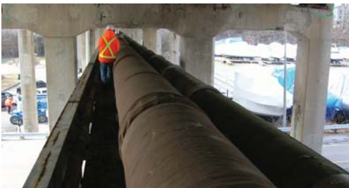
75ft. above a local parking lot the tapes were supplied and the underside applied by an operator on a lift truck.
