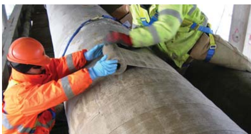
Denso LT Tape was applied in a short amount of time to concrete pipe, providing reliable protection.
