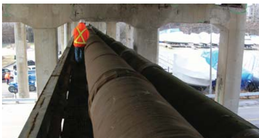
75ft. above a local parking lot the tapes were supplied and the underside applied by an operator on a lift truck.
