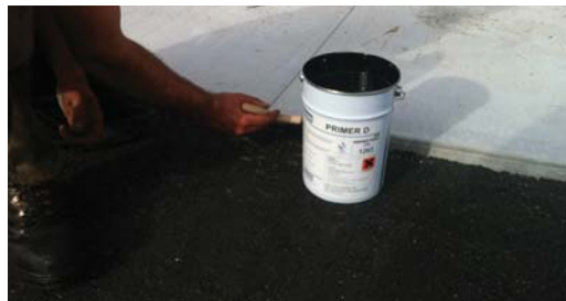
Denso Primer D, a bitumen primer, is applied to the concrete prior to installing the DensoBand along the joint.
