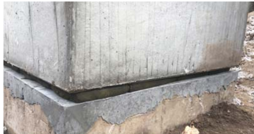
Densyl Mastic is laid upon the prepared surface in preparation for the box chamber.
