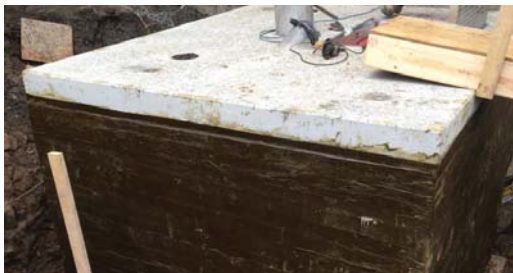
Hi-Tack Paste and Tape applied to the entirety of the structure to prevent water ingress and infiltration.
