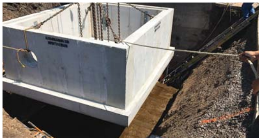
Chamber being set on pre-laid Hi-Tack Tape strips for waterproofing of the base.
