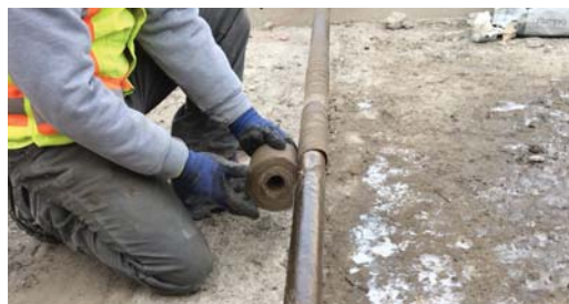
Denso Petrolatum Tape is spirally wrapped, with a 55% overlap, to complete this corrosion protection system.
