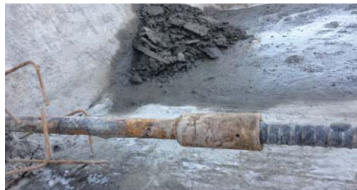
Support rod of the shoreline wall is exposed during the reconstruction phase.
