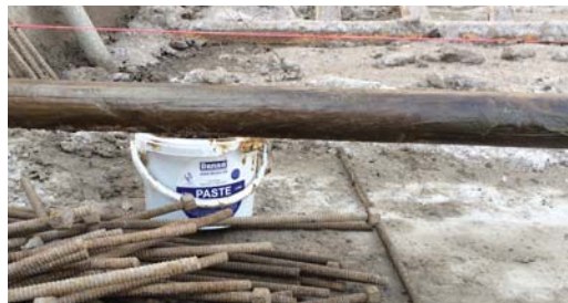
A thin layer of Denso Primer is applied to the exposed substrate prior to the application of Denso Petrolatum Tape.
