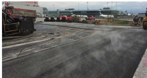
Repaired patch where the DensoBand will withstand future asphalt movement and thermal expansion.
